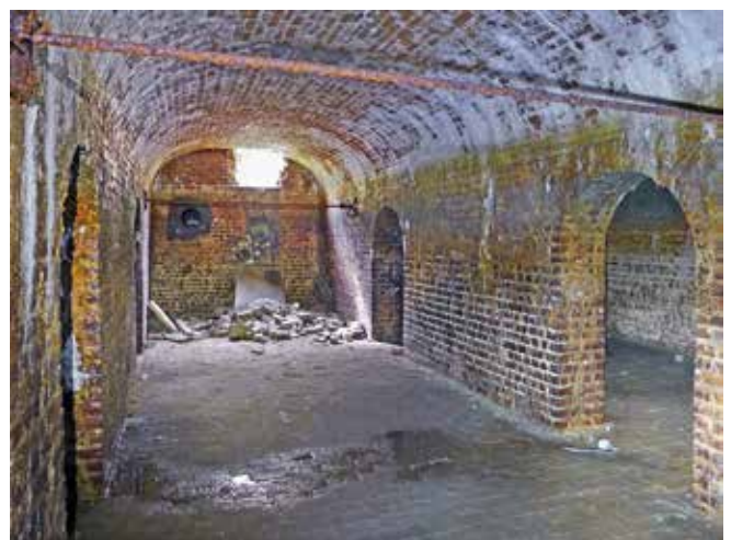
The second chamber with supply pipes (?) in the end wall; the first chamber is to the right
